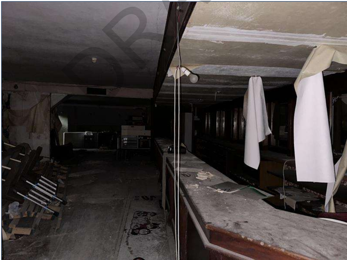
Plate 5-2 Inside of the derelict building at 102 Main Street, Portlaoise.
