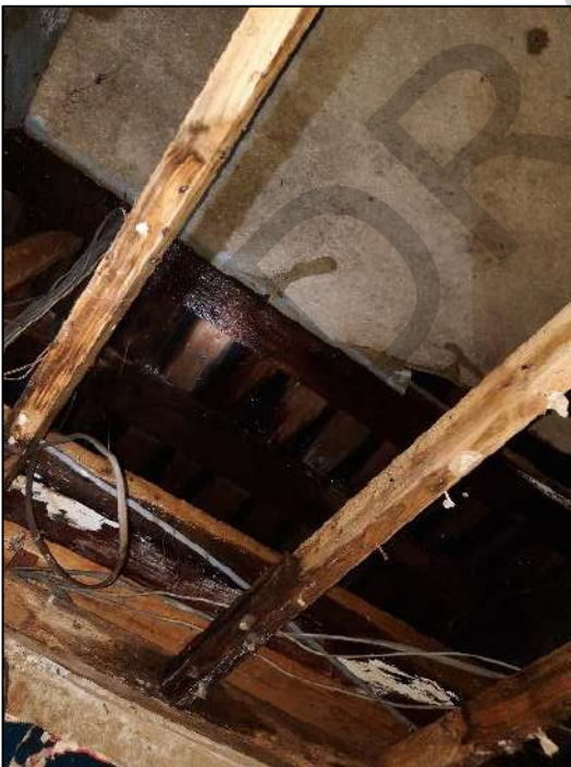
Plate 3-11 Water damage visible of the ground floor ceiling.
