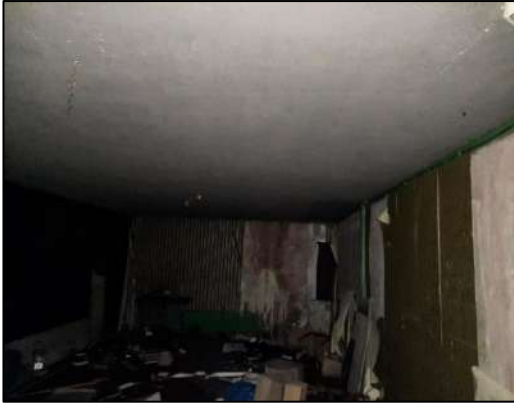
Plate 3-7 Interior section of derelict structure with water damage visible on the walls.
