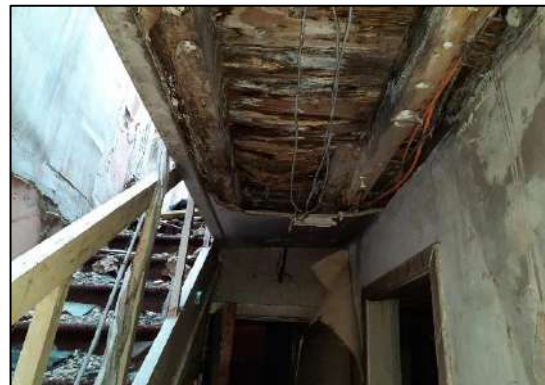
Plate 3-6 Partially collapsed roof with water damage visible within the building.
