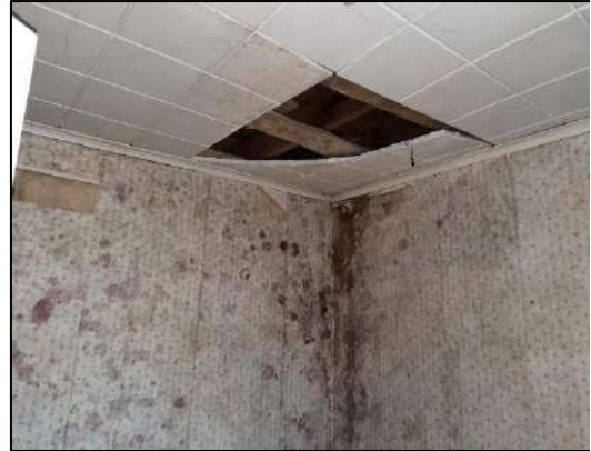
Plate 3-8 Gap in the ceiling with potential access to attic space.
