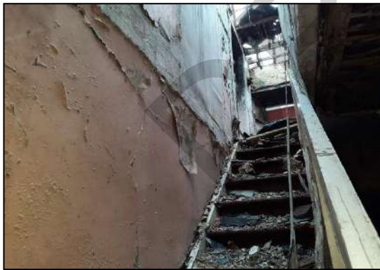
Plate 3-5 Partially collapsed roof with light penetration into building.
