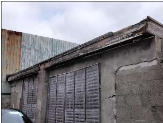
Plate 3-3 Exterior rear view of derelict structure, eastern aspect.
