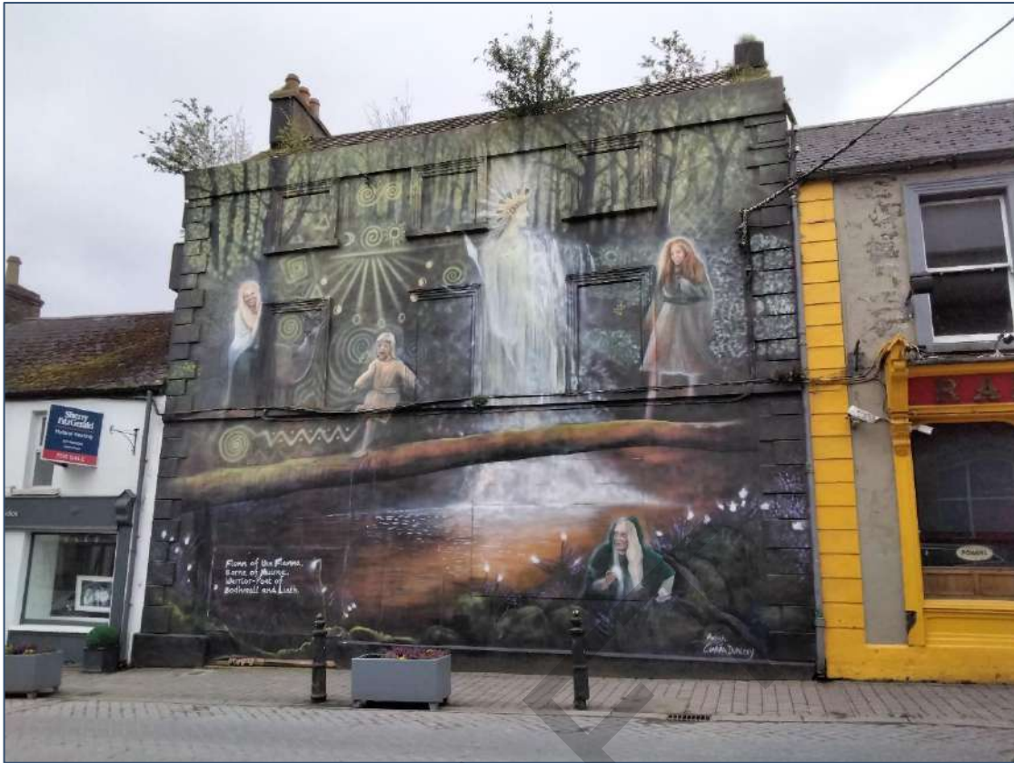
Plate 5-1 Outside of the derelict building at 102 Main Street, Portlaoise, with stands of Buddleia growing from the roof.
