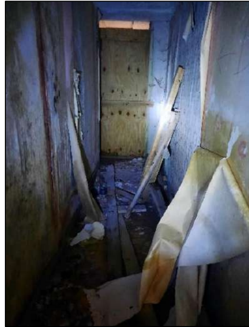
Plate 3-14 Hallway with water damage leading the rear of the property.
