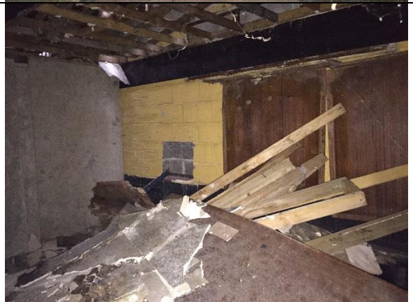
20. Ground floor rear lounge with roof partially collapsed.
