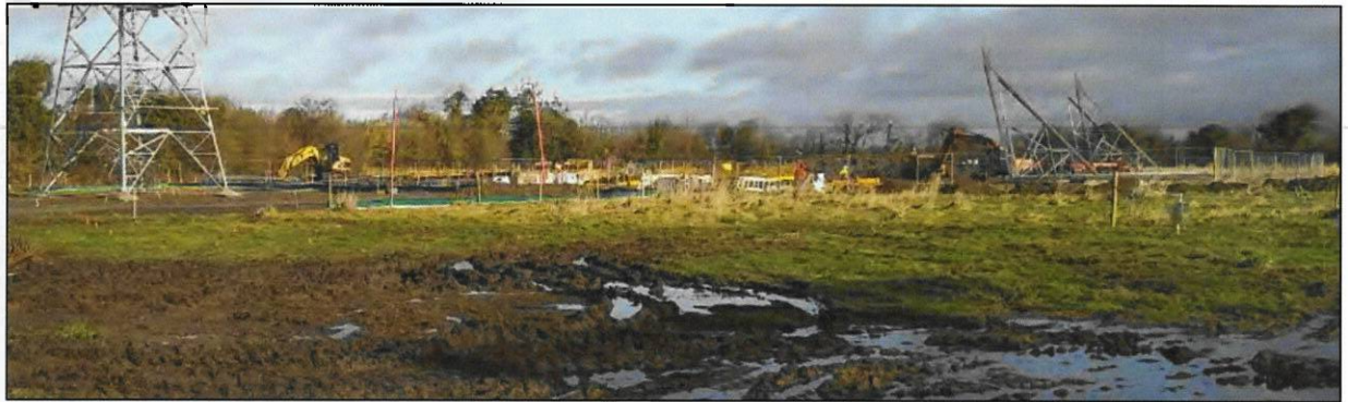
Plate 5 View of Fenced Construction Area associated with 400kV mast works – looking northeast from hard-stand parking area
