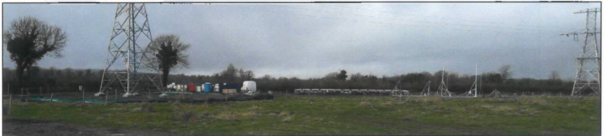
Plate 4 View from Substation Site Area looking west with temporary hardstand carpark in background and new masts to left and right
