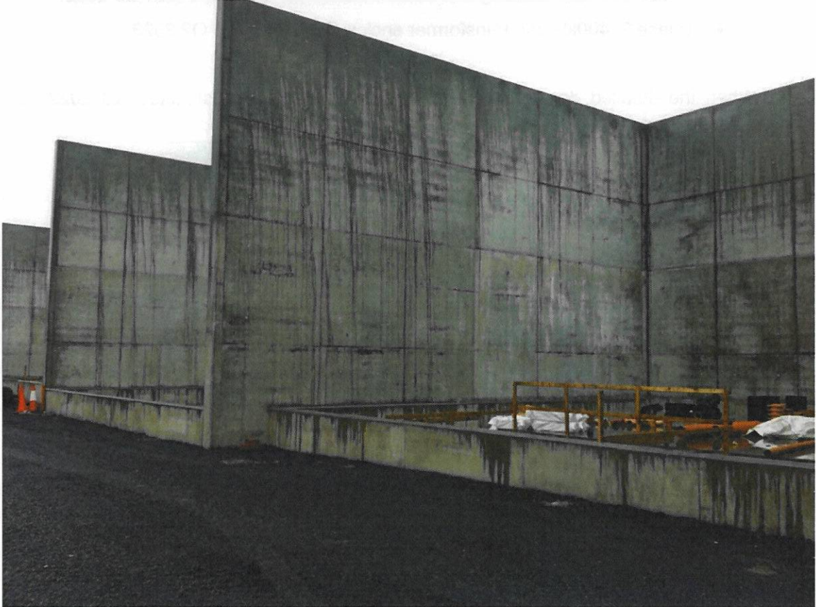
Figure 2.18 Typical walled enclosures for transformers and shunt reactors
