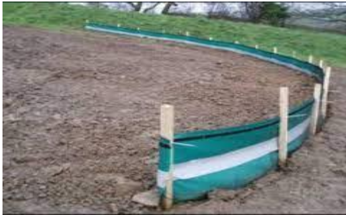
Figure 02 - Example of Silt Fencing
