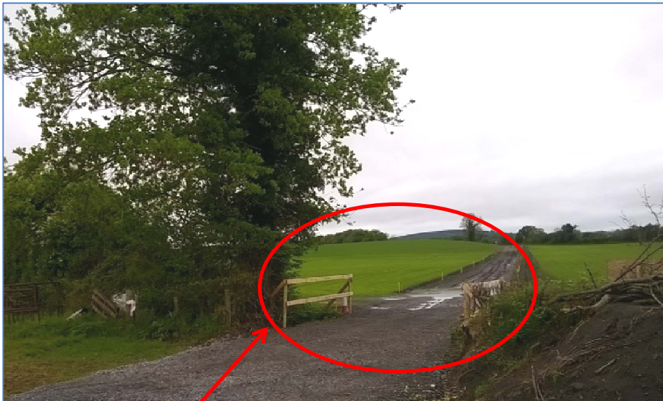
Photograph 3 Dry drain crossing following unauthorized works.
