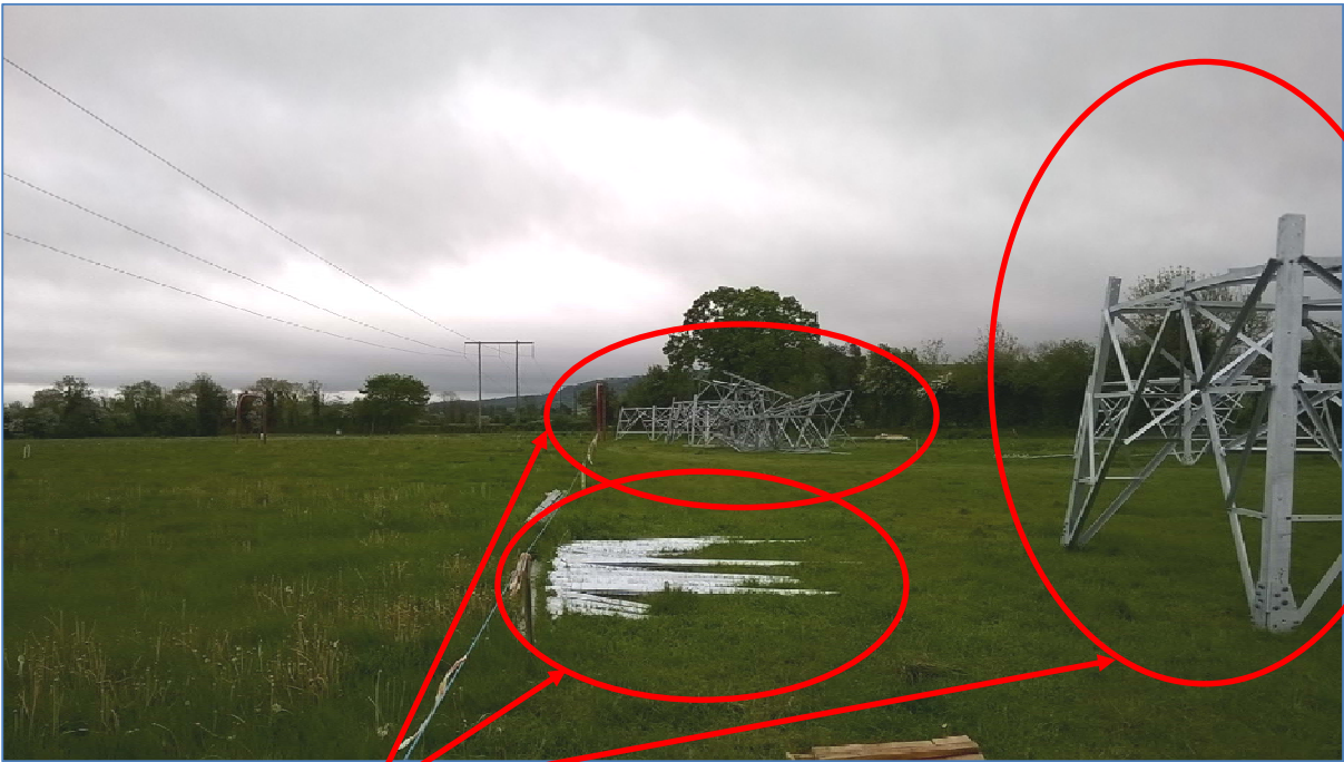
Photograph 2 Materials retained on site following unauthorized works.
