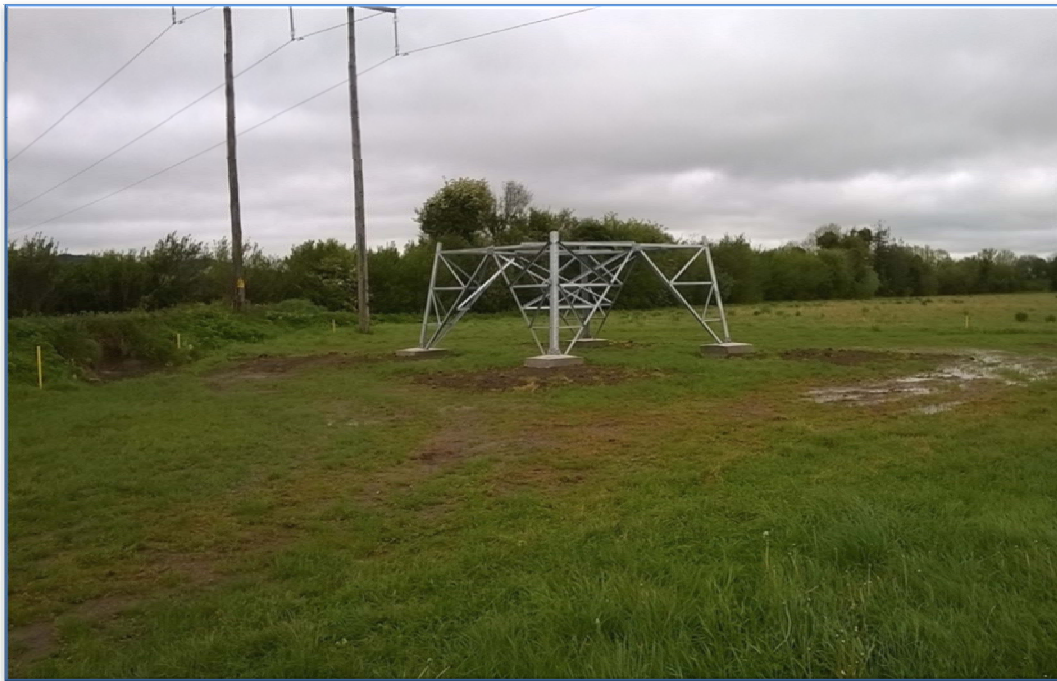
Photograph 1 Tower foundation following unauthorized works.
