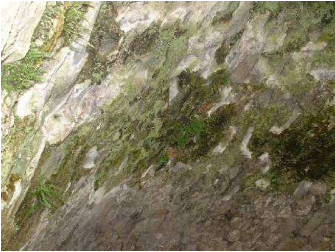
Figure 48. Underside of the Old Stone Bridge (BL1B) supporting ferns, lichens, liverworts and possibly bats.
