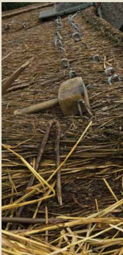
This mallet will be used to rethatch the worn out roof shown here. The straw has become discoloured with age and the hairpin scollops are sticking up. The straight scollops in this section of the roof have been removed, prior to thatching.
