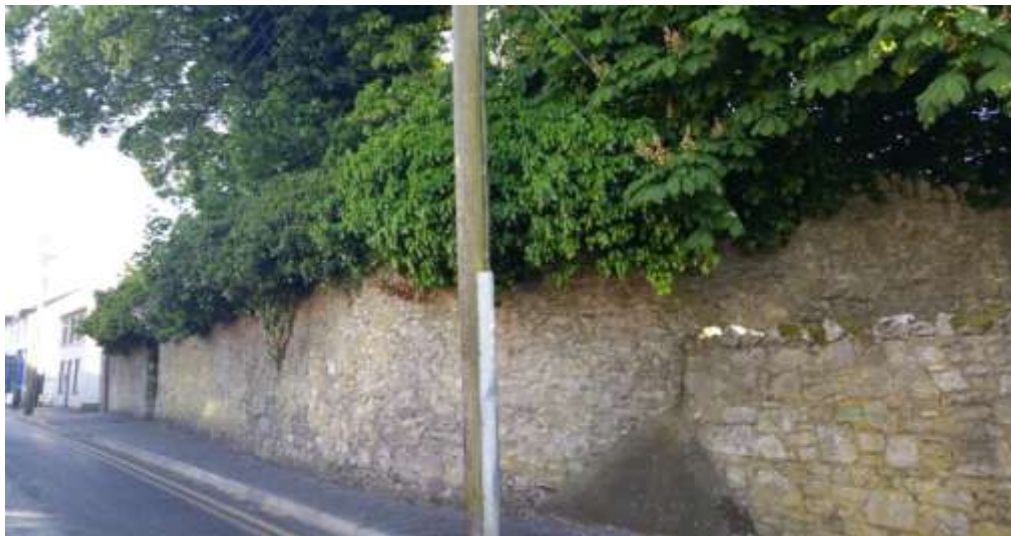
Plate 9: External E wall of graveyard overgrown with vegetation
