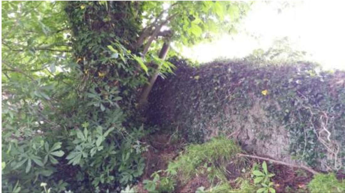
Plate 13: Damage to N wall from mature tree
