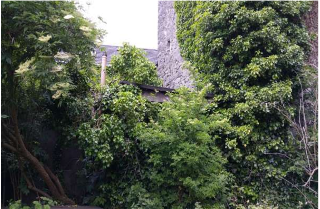
Plate 15: Dense vegetation at base of Church Tower
