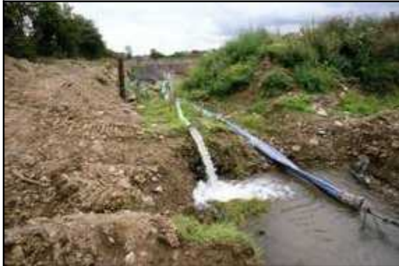
S110_01 Water pump at east end of watered section.
