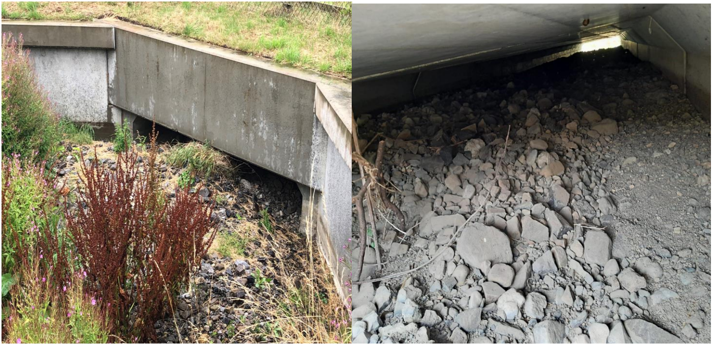
Maidenhead Culvert (Coolanowle Stream) Before Removal of Deposited Material
