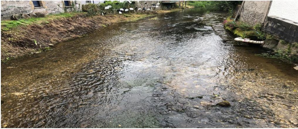
Vacuum Silt Removal Works Completed at Stradbally River at N80 Bridge, Stradbally
