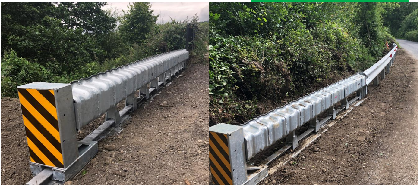
Two new vehicle restraint barriers installed on the L-7894-0 at The Strand
