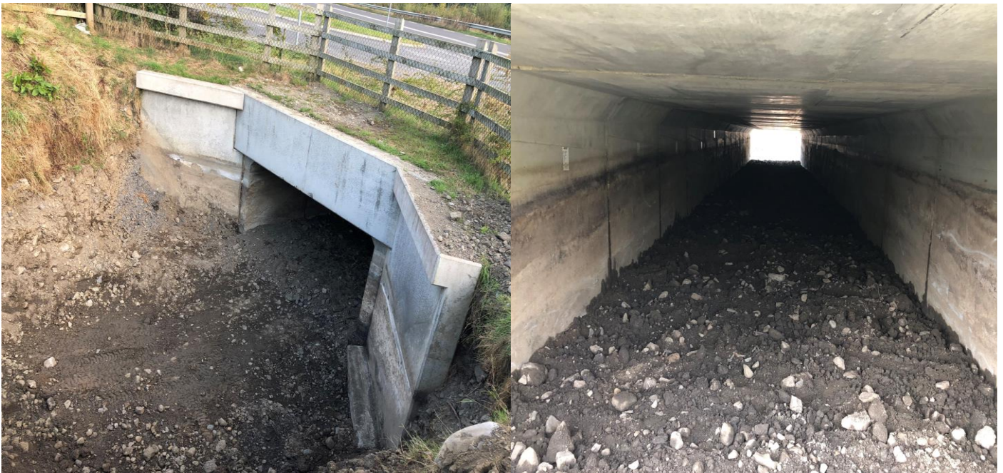
Maidenhead Culvert (Coolanowle Stream) Following Removal of Deposited Material
