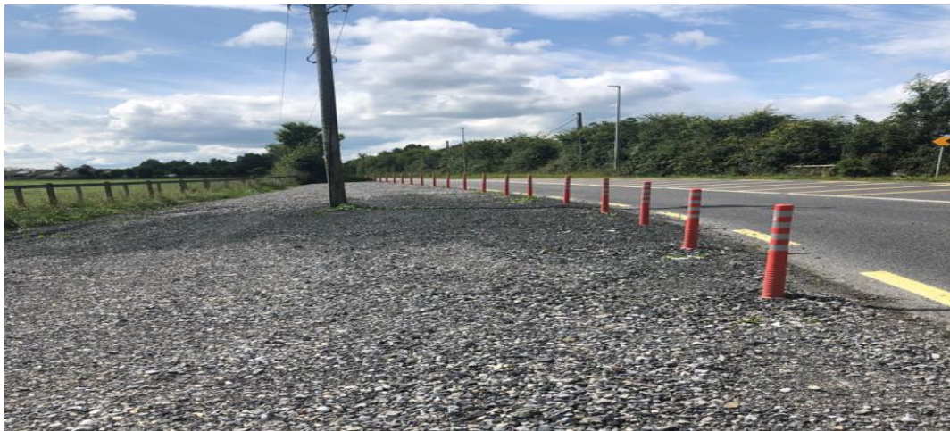
New Safety Improvement Works Completed at the R420/R424 Junction, Lea Cross, Portarlinton
