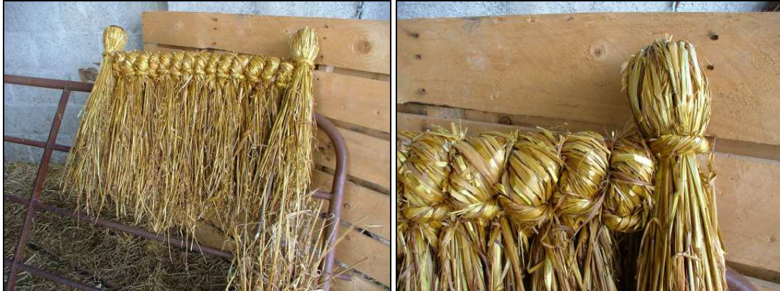
Details of twisted bobbins and end knobs as produced by Mr Michael Dempsey of Abbeyview Cottage, Jamestown, Ballybrittas. Mr Dempsey finishes a ridge using this method.
