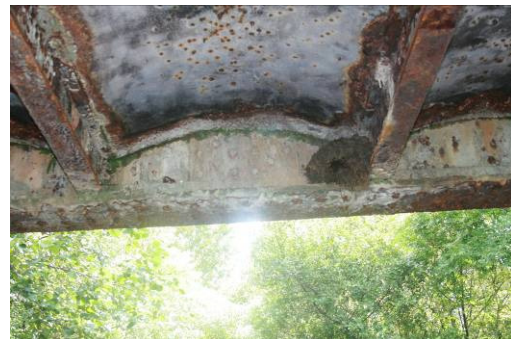
Fig 1.2 Dipper nest on girder flange Lacca Bridge, Delour River
