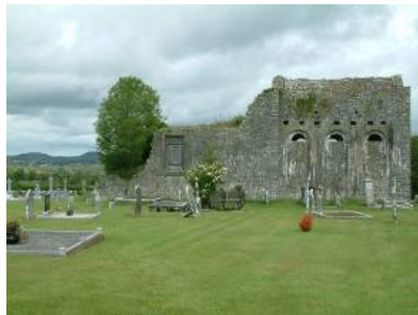
Ash tree growing on top of the southern wall of the nave, looking north
