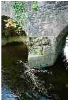
LAIAR-016-007_03 FWH 30/08/2007 Damage caused by shrub to upstream river cutwater.
