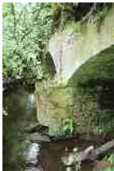
LAIAR-017-004_03 FWH 14/06/2007 Upstream pier and cutwater at west end of middle arch.
