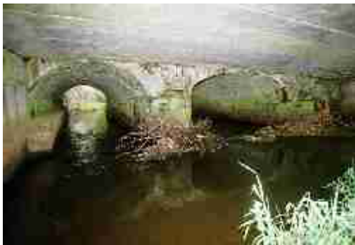
LAIAR-021-008_03 FWH 31/08/2007 Upstream elevation showing left and middle arches and later addition.
