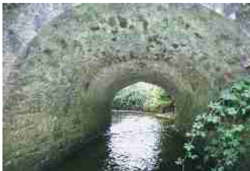
LAIAR-035-009_03 FWH 28/09/2007 Break in soffit, looking downstream.
