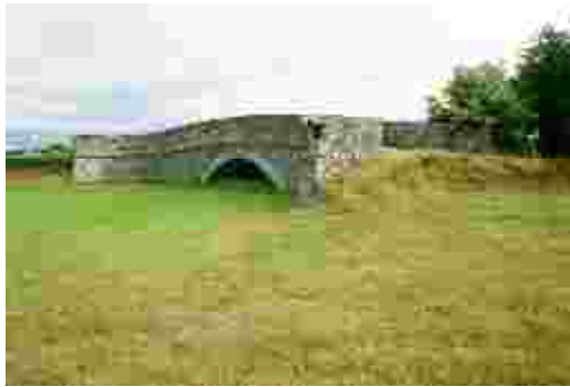
LAIAR-008-030_01 FWH 29/06/2006 Skeagh Bridge from south-east. Note damaged pier at right and removed approach road.
