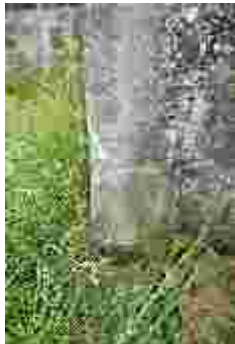
LAIAR-004-010_06 FWH 29/06/2006 Tow rope marks on east quoin.
