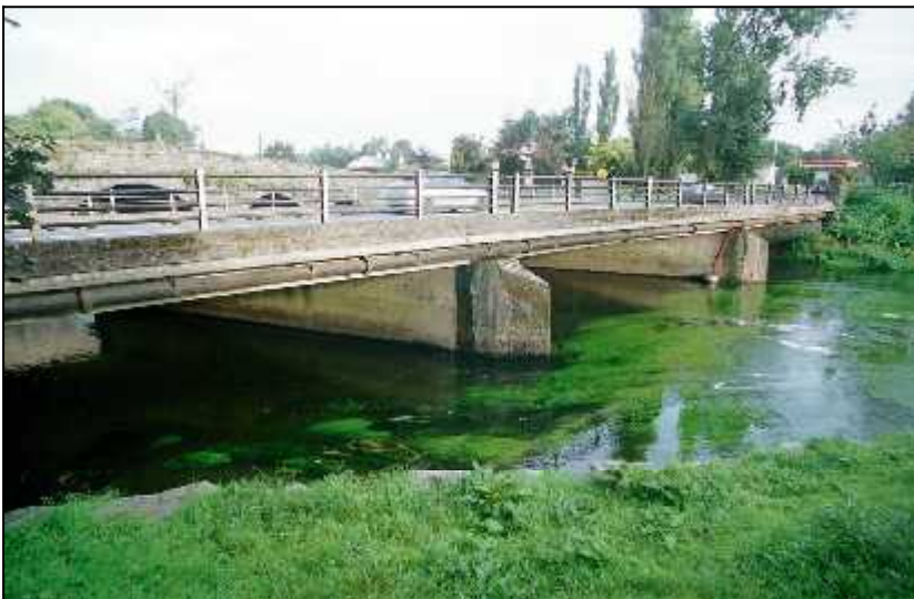
Fig 3.34 Pre-cast reinforced-concrete beam and slab triple-span bridge over Erkina on the main N8 at Durrow (029-046).
