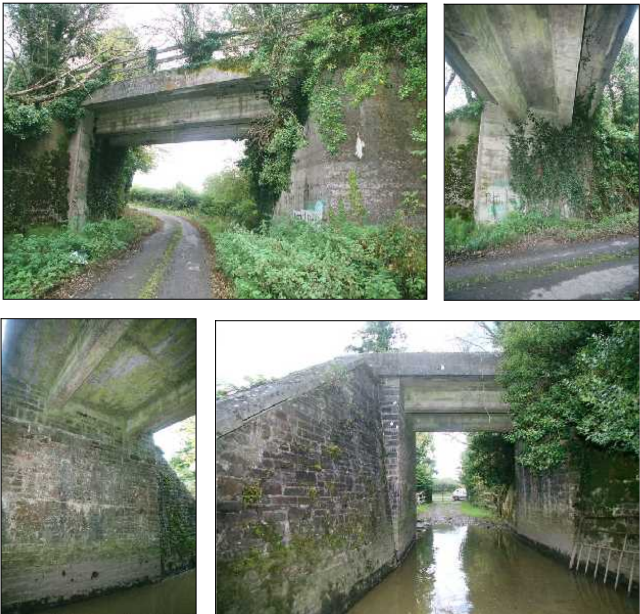
Fig 3.28 Concrete bridges at Kilfeacle on the Wolfhill Line. Top : Bridge over public road, with skew span and concrete abutments (025-023). Bottom : Orthogonal span over accommodation road (025-028). Unlike the previous bridge, its abutments and wing walls are of rubble masonry.
