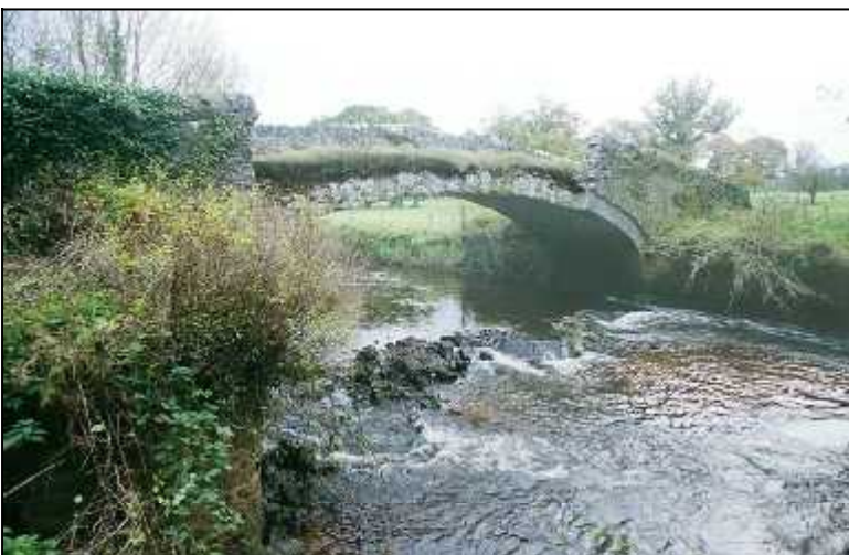
Fig 2.5 This accommodation bridge over the Nore in Abbeyleix Demesne has the longest masonry arch span in the county (029-005).
