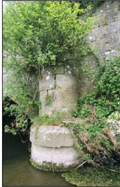
Fig 6.6a Far left : Undermining and partial collapse of upstream cutwater at Rushin Bridge over the Mountrath River (017-004).
