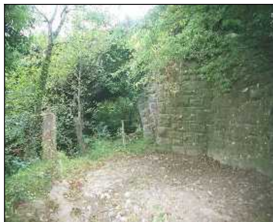
Fig 6.10 The deck of this bridge at Grenan, on the Kilkenny border, is now inaccessible and almost completely overgrown with ivy (035-010).
