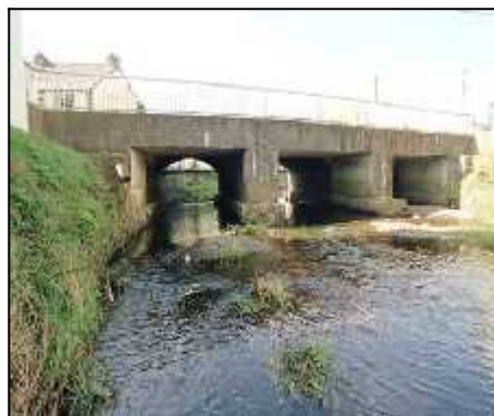
Fig 2.23 Upstream (left) and downstream (right) views of Convent Bridge, Mountmellick. The latter is a concrete slab widening of the original masonry bridge (0081-016).
