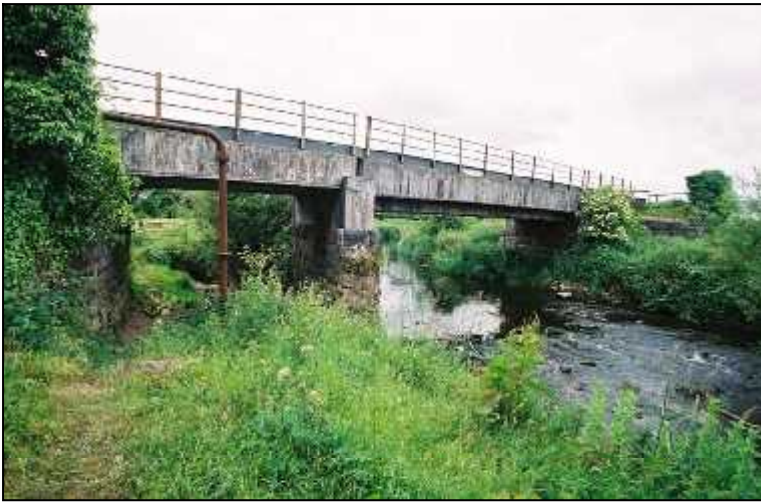
Fig 3.22 This skew triple-span concrete beam bridge carried the railway over the Barrow (004-022).
