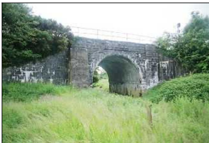
Fig 6.3 Gunited arch soffit on bridge carrying the main Dublin-Cork railway over a tributary of the Nore at Clonadacasey (017-0168).
