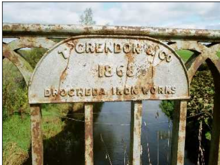
Fig 5.3 This plaque on the modern Derryduff Bridge (016-003) recalled the date of the previous plate girder bridge built by Thomas Grendon in 1868.
