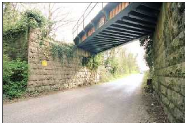
Fig 3.23 This bridge at Cooltedery shows the single-track deck on its double-width abutments (005-005).
