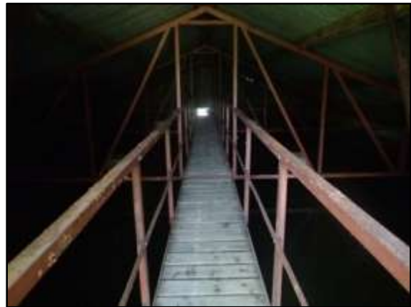
A view inside the galvanised steel hut, where a gangway leads across the spring water.
