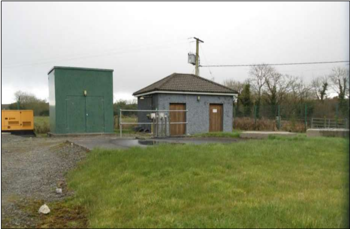
Pumphouse and works at Swan Public Water Supply Scheme. Clogh River to right near trees.
