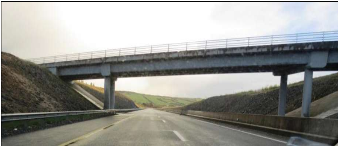
View looking south under bridge carrying local Rathdowney to Cullahill road over M8.
