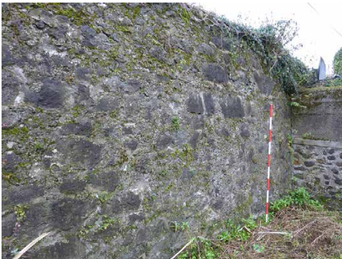
Fig. 100: Detail of exterior of fort wall, showing thin line course, in Site 18 from the south west (Eoin Sullivan)
