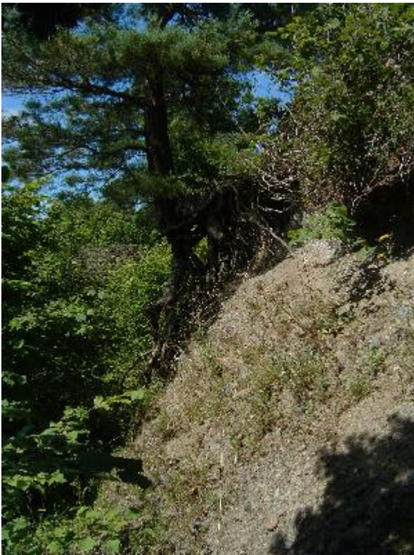
Plate 5.2 Erosion under the Ridge Road
