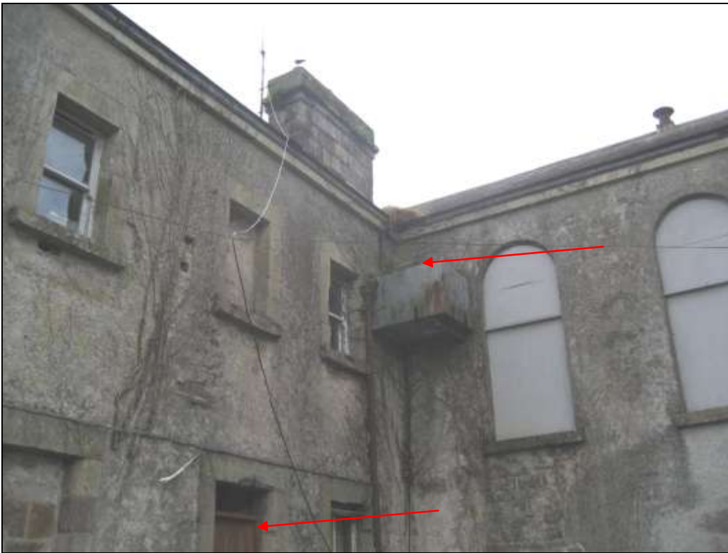
Figure 1.3 Borris in Ossory Courthouse showing gaps in soffit boards and missing glass above the door, which allow access for Pipistrelle and Brown Long-eared bats
