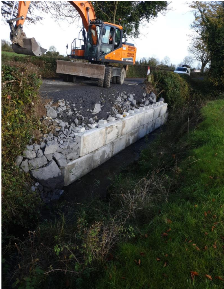
Embankment collapse Summergrove, Mountmellick
