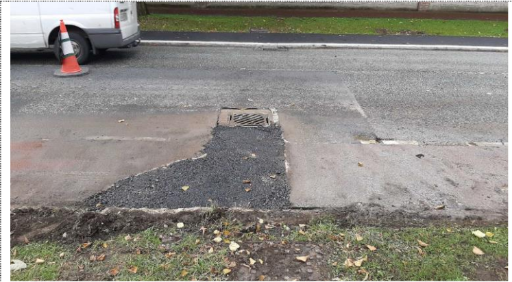
Step 2 Temporary tarmac to new gully pot, notice the road narrowing intentions
