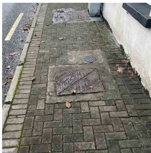
Poor quality surface finishes
