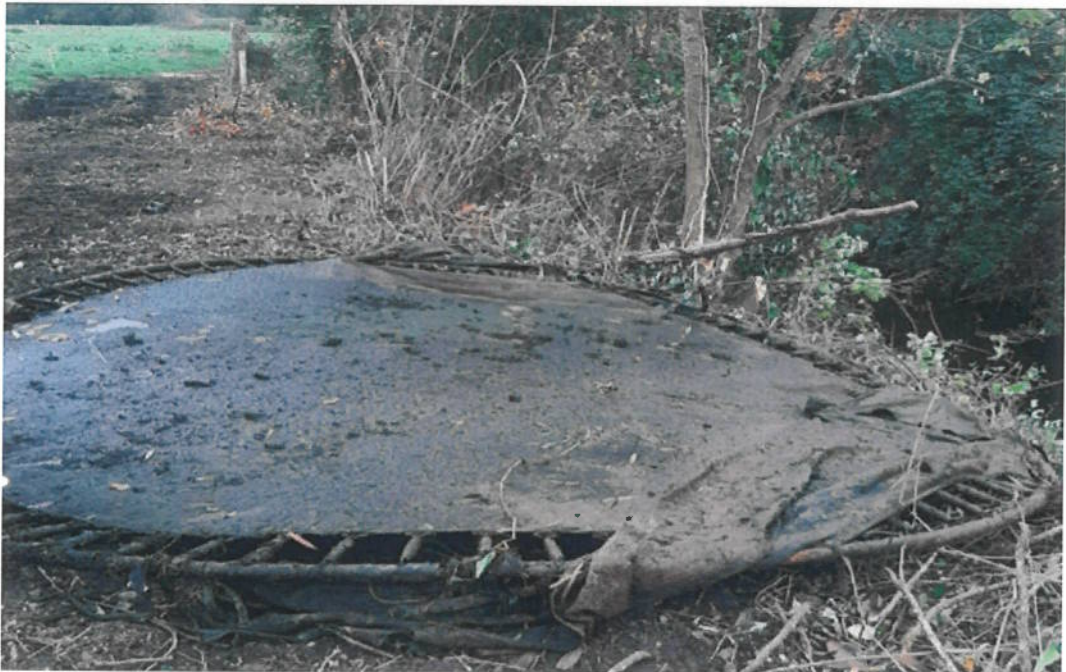
Stradbally River (trees encroaching into river and fallen trees) ~ After
