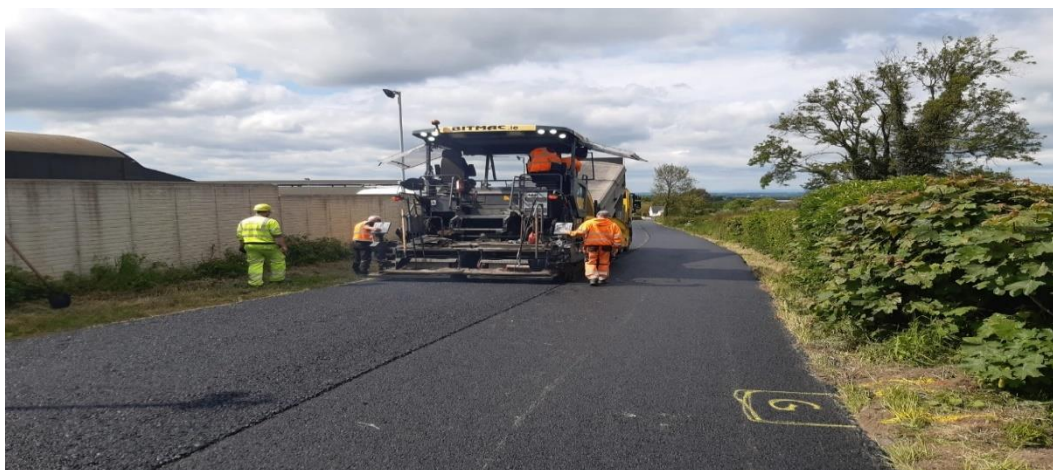
Works commenced on Restoration Improvement Programme in Portlaoise Municipal District in Cloncullane, Ballyroan
