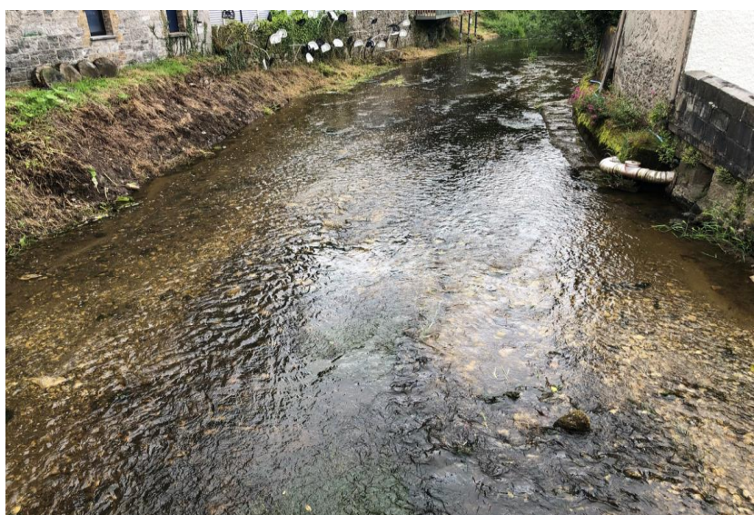
Vacuum Silt Removal Works Completed at Stradbally River at N80 Bridge, Stradbally
