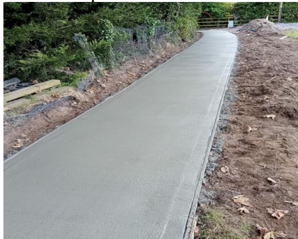
New Footpath from Timahoe National School to Hillview- Works in Progress July 2024
